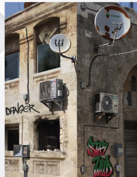
35638 AIR CONDITIONERS &amp; SATELLITE DISHS
